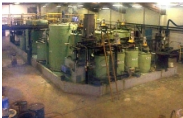
Figure 9: The purification circuit at the Intec Copper demonstration plant, with cupric reduction in the foreground, and pH4 purification in the background
