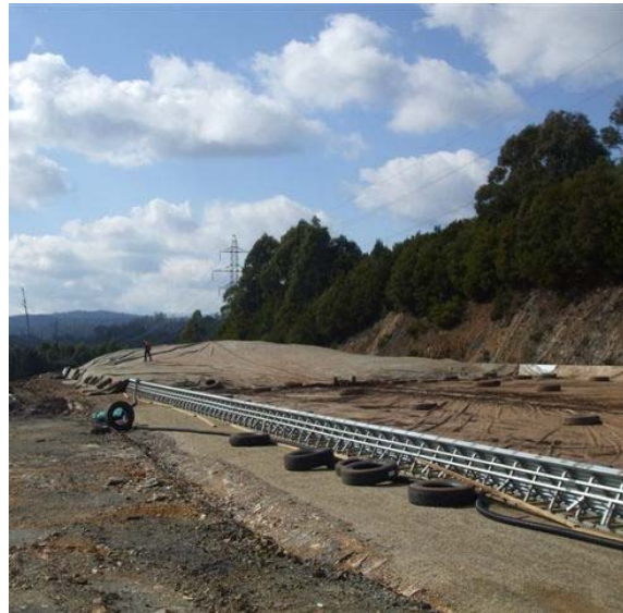
The EAF dust bunker at the Hellyer Residues Project site. Feedstock is stockpiled in a growing pile, ultimately to reach seven metres in height
