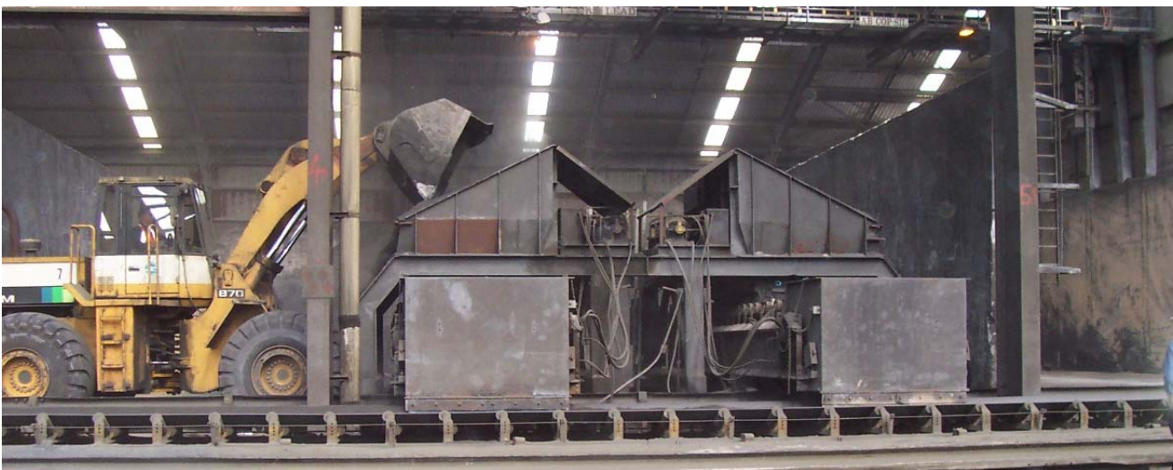
Above – Concentrate being loaded from the HZCP’s storage bay at the Port of Burnie into hoppers feeding the conveyor belt on to the “M.V. Mount Rainier”
