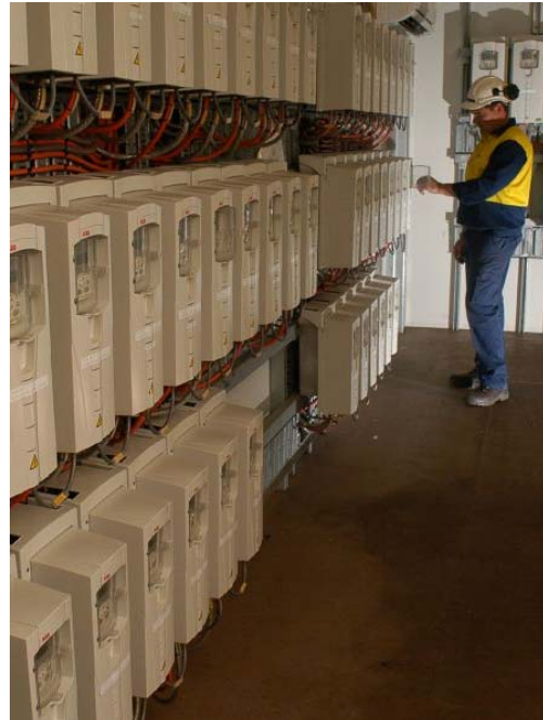
An operator in the motor control centre of the Burnie Demo Plant
