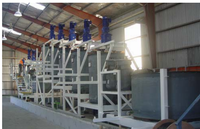
Figure 1: View of the complete leach circuit now installed in the Burnie demonstration plant. The base metals leach (including two leach tanks and thickener) is at the far end of the building, with the pyrite leach (including five leach tanks and thickener) in the foreground. Mixer drives are in place on top of each leach tank.
