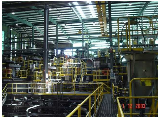
Figure 5: Partial View of Flotation Circuit at Hellyer
